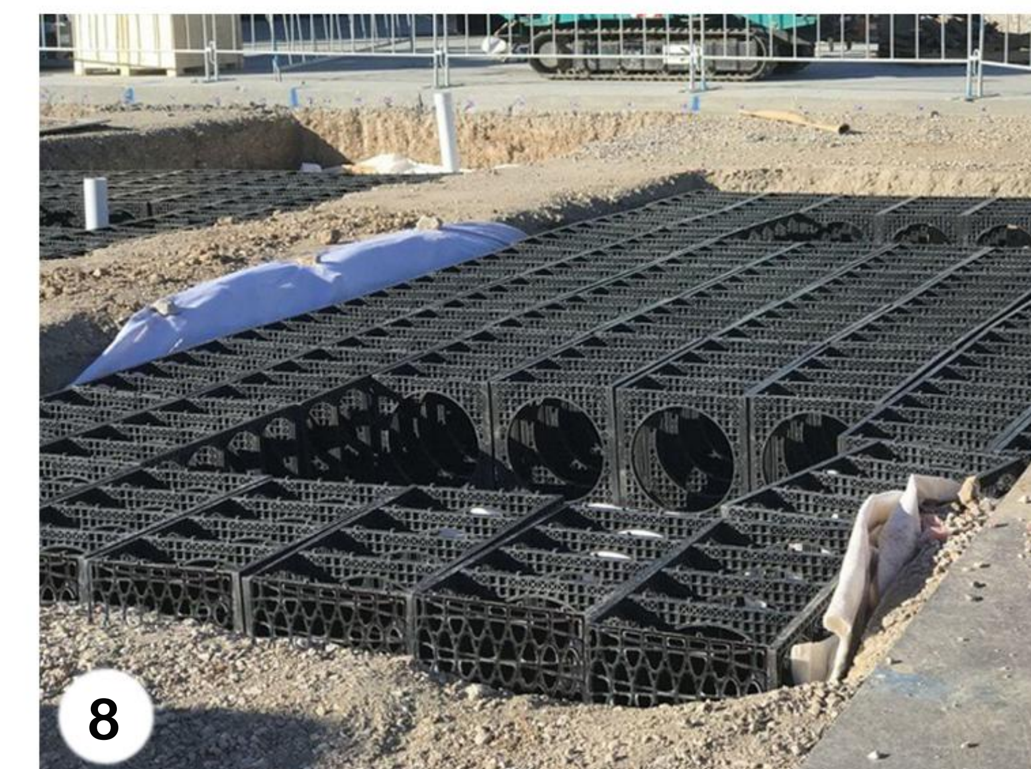
8 Add the crates to your excavation with the open tops. Fill modules with nutrient-rich soil. You can then attach the final Ellipse large closed plates on top of the modules.
